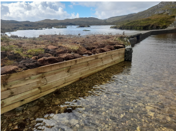
Connecting new part of Urgha loop walk across Lochannan Lacasdail to the original path. This was to reduce erosion on bank edges and the bridge.
