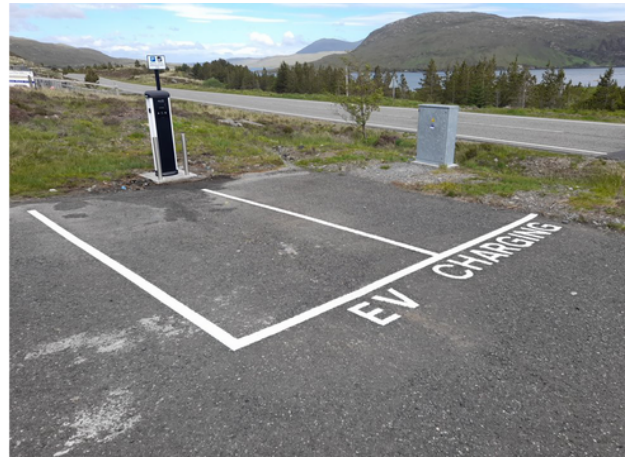
Electric Vehicle charge point installed as part of Àird Mhulaidh.
