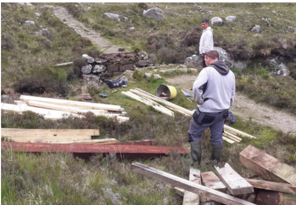
Replacing the first bridge as you ascend the Abhainn an t-Sratha from Urgha as main beams were rotten.
